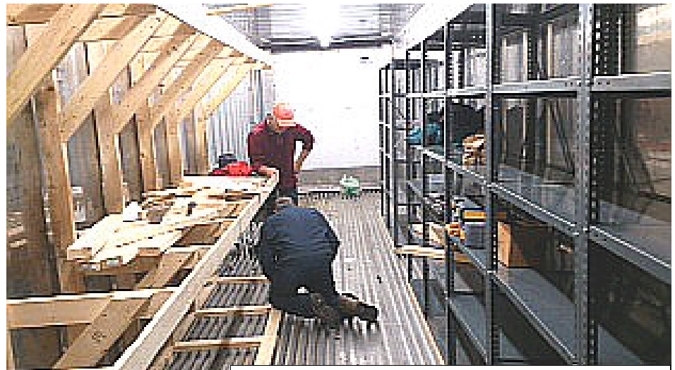
Work in progress - John, VE1CDD, downed tools long enough to photograph Fraser, VE1WO, and newly licensed Bill Hebb, VE1HEB, "customizing" the HARC's new storage facility
