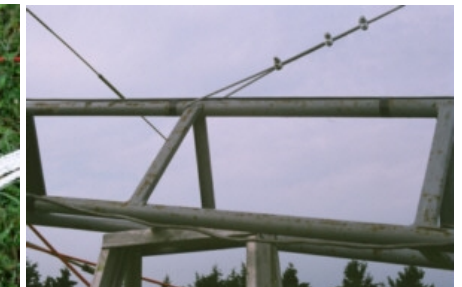
The top of the derrick is wire-roped to a point part way up the tower
